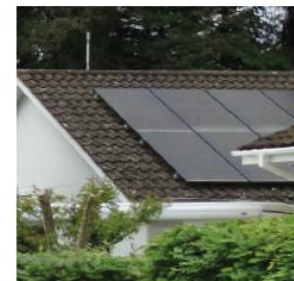
Roof solar panelling.
